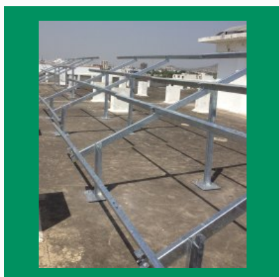
Solar Panel Mounting Structure
