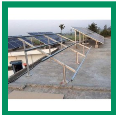
Solar Mounting Structure
